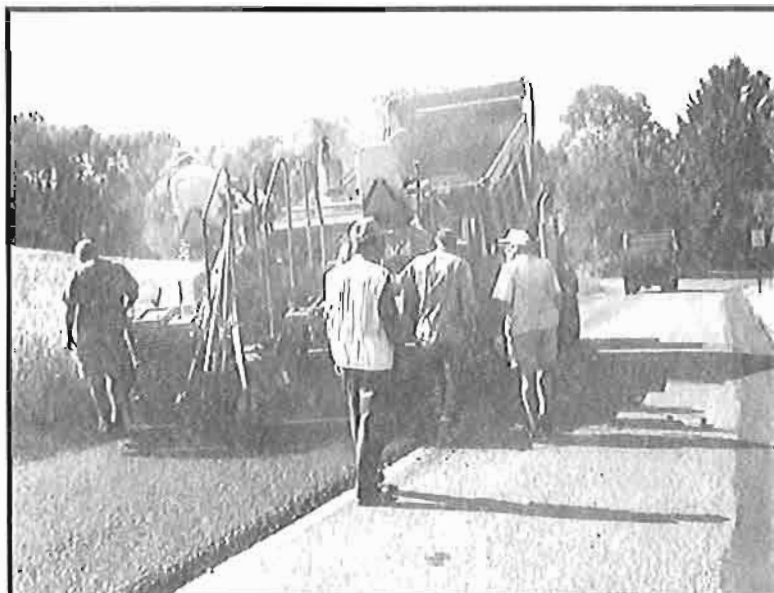
Supervisor Ron Stahley confers with a member of the contracted paving crew as they pave a portion of Rockdale Road.
