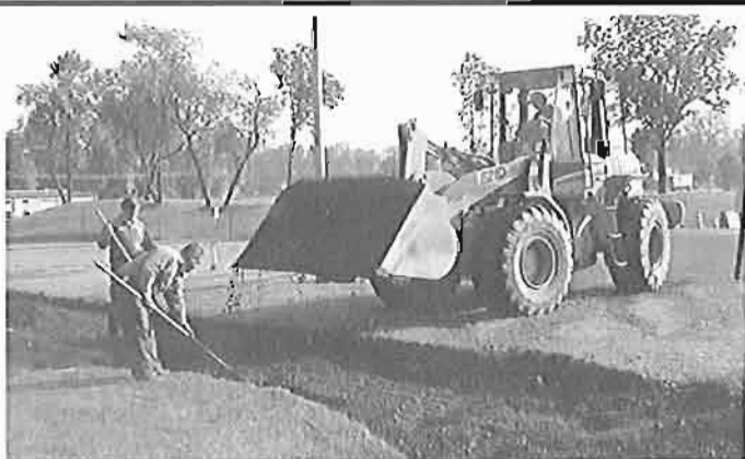
Loader operator Dave Crilley places stone for Doug Wetzel and Kris Kreglow as they work on a new walkway.
