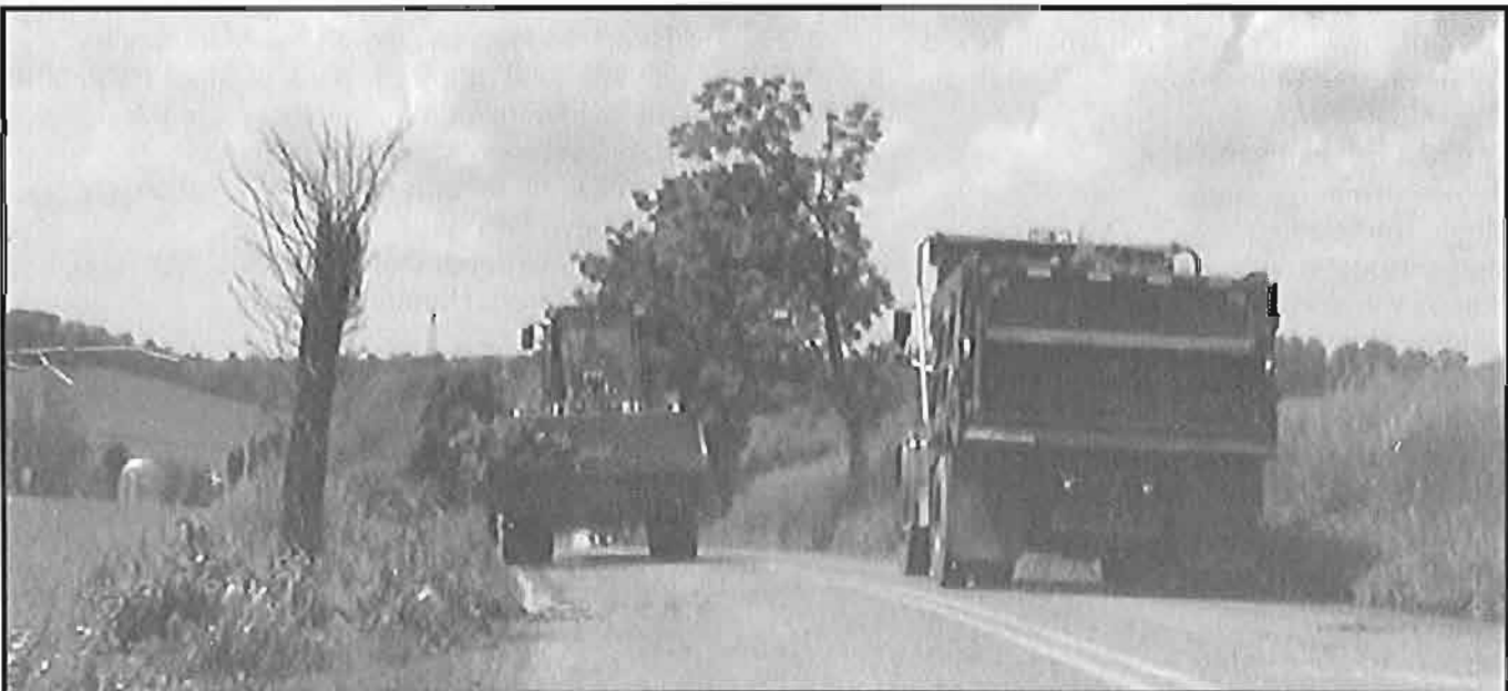
Tim Trunk and Gary Kressley clear road shoulders on Hillside Rd. in preparation of bituminous seal coating.
